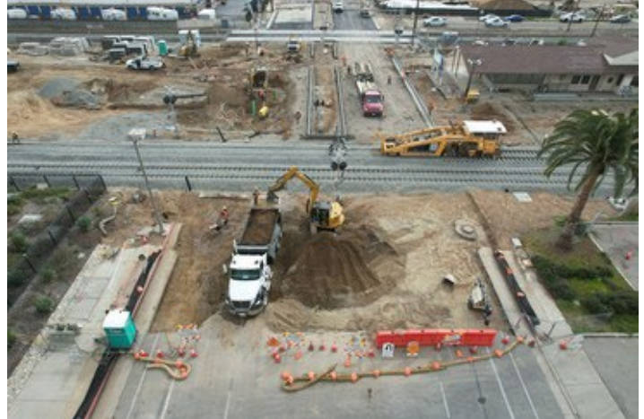
View south of the Garey Avenue crossing in Pomona on the Foothill Gold Line extension, the last crossing to be rebuilt.
