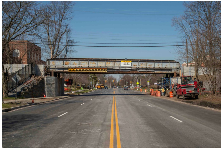
Compare this view, taken after the third weekend “lift,” on March 21, with that on page 5 in last month’s Bulletin. You can see how the bridge has been raised above the tops of the abutments on each side.
