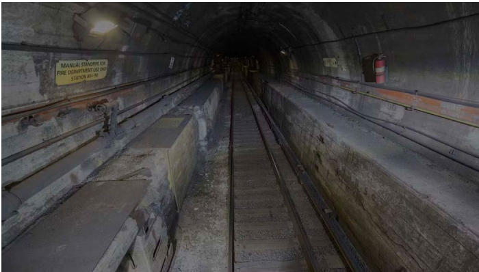
The interior of one of the tubes of Amtrak's East River Tunnel, which was originally opened in 1910 and sustained damage during Superstorm Sandy in October 2012. Amtrak photo
