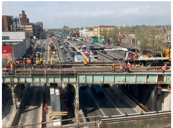
View north of the old Main Line bridge carrying Tracks 3 and 1 over the Van Wyck Expressway as seen on April 16. Jeff Ertlitz photo
