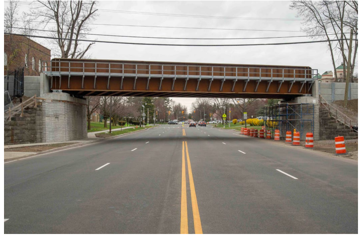
Looking north on Cherry Valley Avenue in Garden City on April 7 with the new bridge now in place. The old bridge was dragged off to the right of this image to the location where this new bridge had been assembled. Jeff Erlitz photo
