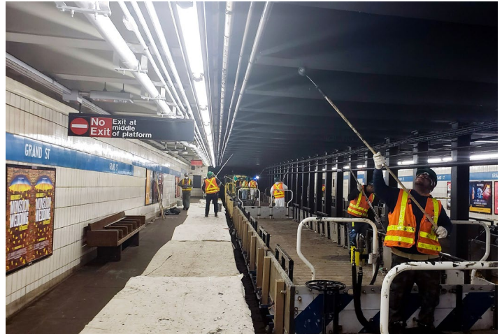
Grand Street station during the Re-NEW-ation work over the weekend of 15-16. Aaron Donovan/MTA photo
