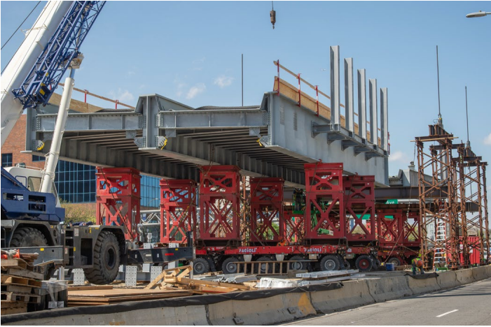
The new bridges were assembled between the Van Wyck's northbound main and service roads, two blocks north of the railroad, just south of 90th Avenue. This is looking north from the sidewalk of the northbound service road on April 19. Jeff Erlitz photo
