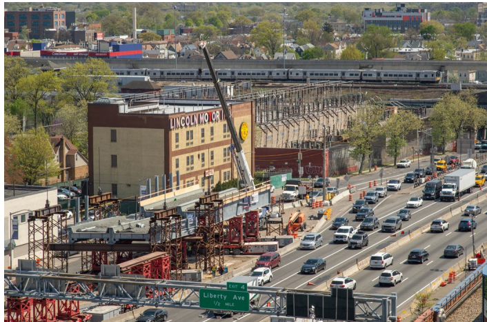
An unusual view from the parking garage of Jamaica Hospital of the new bridges. In the distance, M7 7167 (Bombardier Transportation, 7/2003) and train #2911 has just left Jamaica station and is beginning its shuttle trip into Brooklyn. Jeff Erlitz photo
