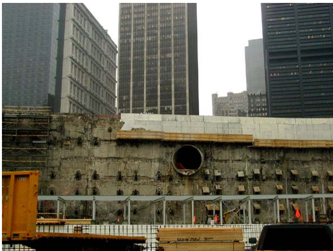
Old Hudson Terminal Tube seen above new steel for World Trade Center temporary station.
