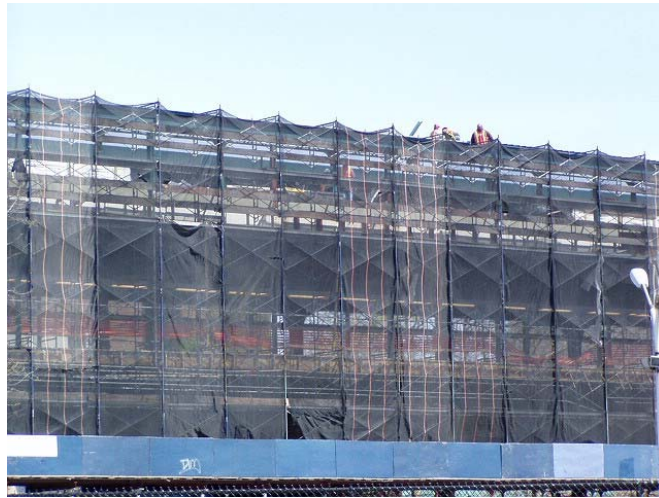
All dressed up with no trains to roll...the W. 8th Street station under reconstruction.
