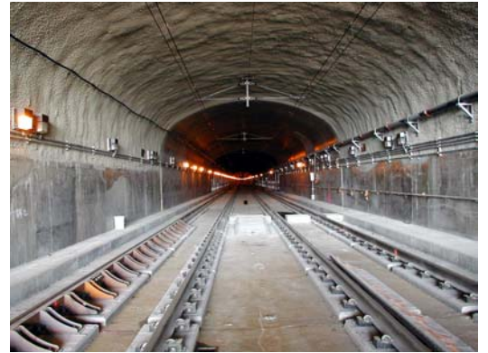
Tunnel section inside the River Portal, showing shotcreted section of the roof (formerly brick lined).
