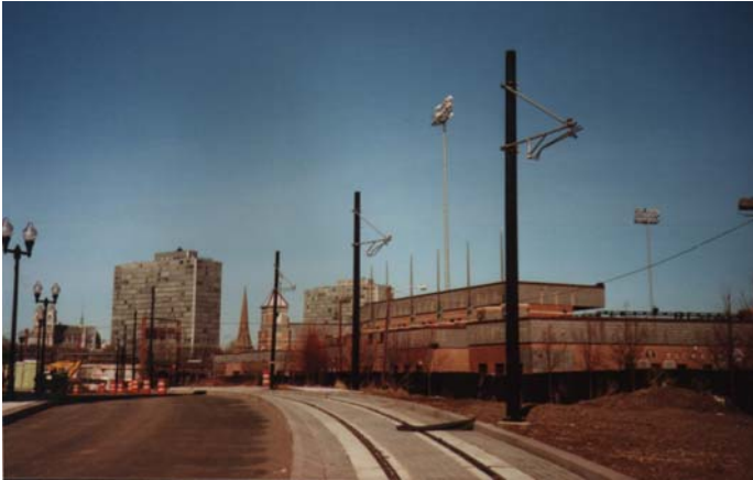
Single track (northbound) approaching Broad Street station. Wire about to be installed.
