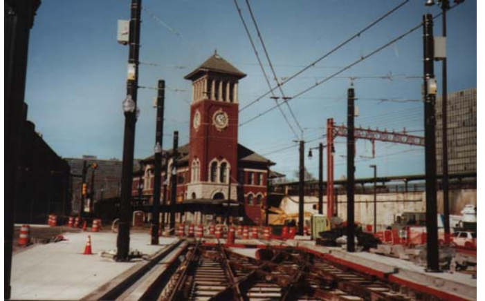
Construction in front of Broad Street Station, terminus of the 1.3-mile extension.
