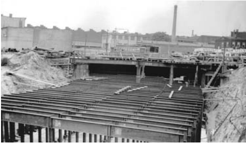
Fulton Street Subway construction in May, 1940. Car 1176 crosses on the Jamaica Avenue line.
