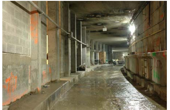
Looking north on Track 4A north of the station. The double crossover is located roughly 300 feet north of the platform, just beyond the slight curve in this view.
