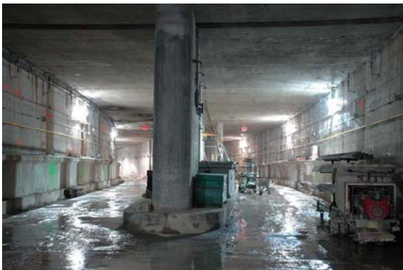
Looking south at Tracks 4A and 1A from the location of the future double crossover.
