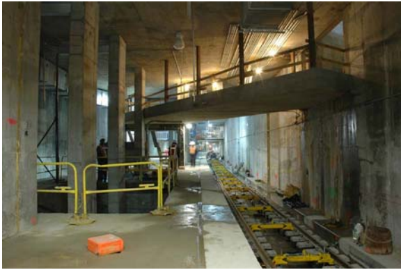
Looking north on Track 4A (northbound side) at the south end of the platform. The passageway to the Staten Island Ferry terminal can be seen above the track.
