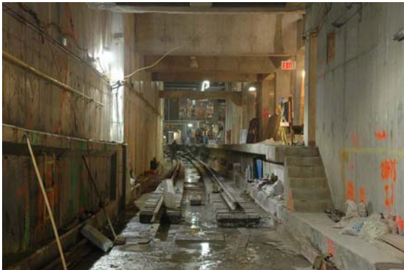
Looking south on Track 4A at the north end of the platform. The skeletonized Type II track has already been installed and is awaiting the concrete pour. This is the only track installed so far.
