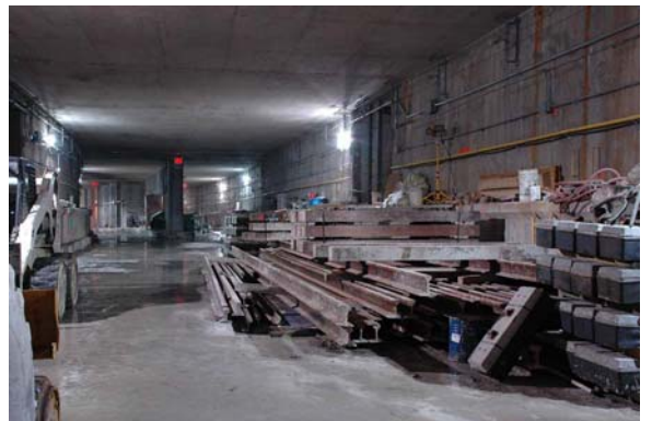
Looking south at rails and half ties temporarily stored in the area of the future double crossover.
