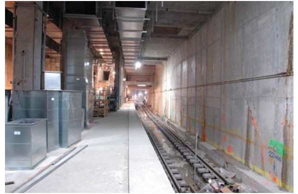
Looking north about 200 feet south of the north end of the platform. A lot of the ductwork for the air tempering system can be seen both on the platform and up on the ceiling.
