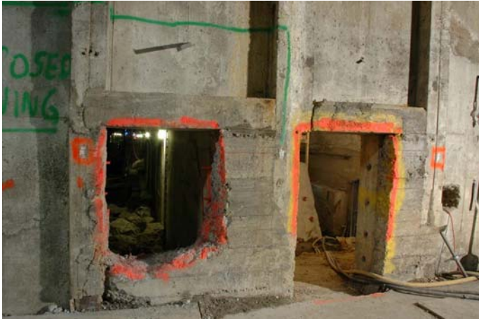
Looking east from the IND 42 nd Street station lower level platform, we see the openings cut into the wall leading to the Flushing Line. Track 1 is on the left.
