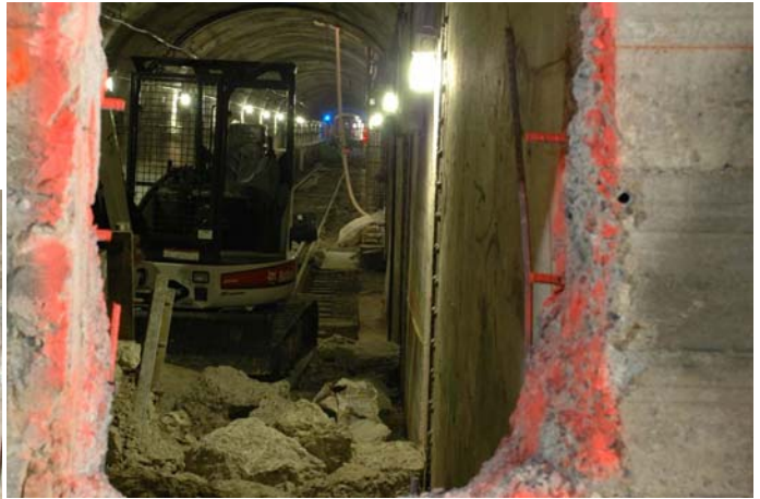
A telephoto view through the opening in the wall shows Flushing Line Track 1 with the Bobcat where the bumping block once stood.
