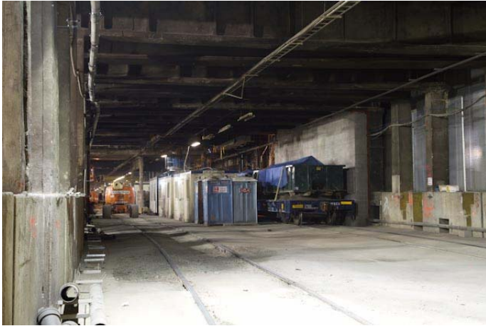
Freight cars being used to haul construction debris before tracks are removed.
