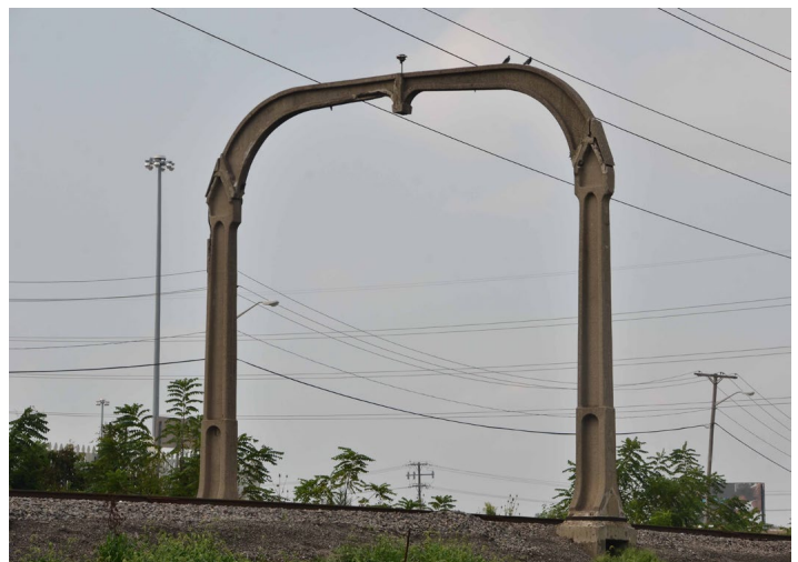
A long-abandoned concrete catenary mast stands outside of Dearborn, Michigan along the former DT&I railroad right-of-way. Installed during the period of Henry Ford ownership and investment, the electrification was only briefly used. After attempts to remove the well-built masts proved complicated and expensive, many such as this one have been left in place and see only the occasional diesel-powered freight trains pass. Photo taken September 1, 2013. Paul Grether photo
