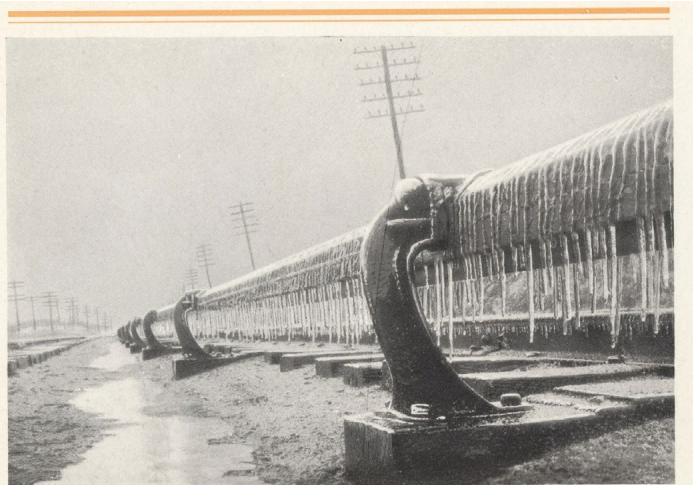
W.-S. UNDER-RUNNING THIRD RAIL DURING SLEET STORM, THE CONTACT SURFACE BEING FREE FROM ICE
