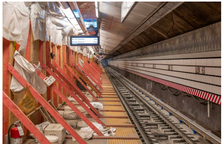
A view behind the construction barrier along Track T1 in Lexington Avenue/63 Street station on March 21. The new Type II-Modified track replaced the original Type VIII track. Jeff Erlitz photo
