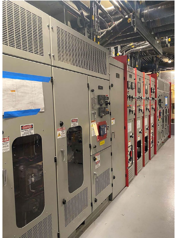
The new substation at Civic Center Station, on May 2. BART photo
