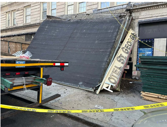
The collapsed awning over the Clark Street 2 3 Station entrance on Henry Street. Steven Vago/NY Post photo
