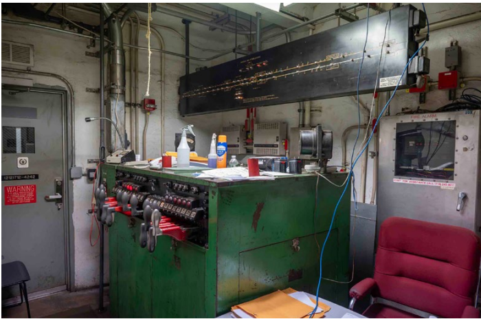
The 24-lever GRS Model 5 interlocking machine in Nassau Avenue Tower, as seen back on December 19, 2024. Jeff Erlitz photo
