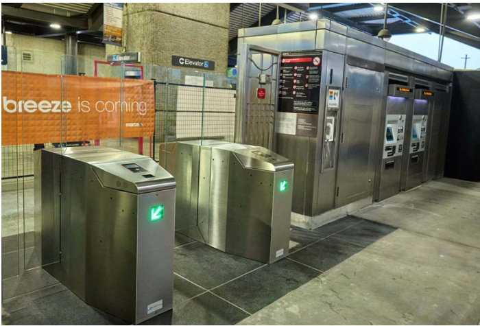
Better Breeze faregates and ticket vending machines at Lindbergh Center Station southeast entrance. MARTA photo
