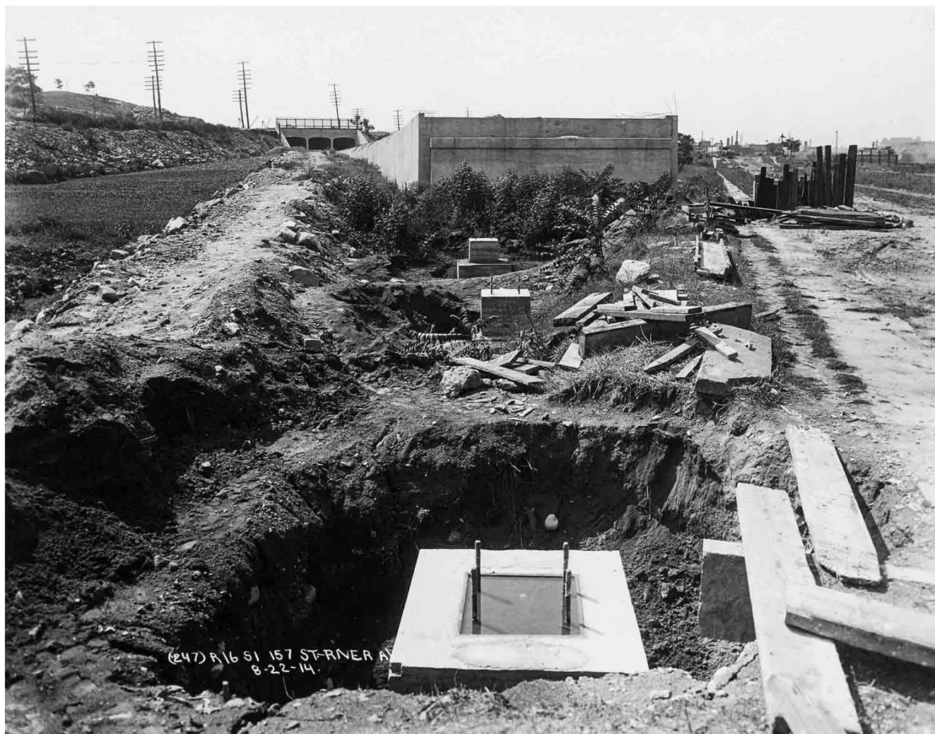
Looking south on August 22, 1914, south of the 161st Street station. This is the earliest view we currently have of Jerome Avenue Line construction photographs and was taken near the southeast corner of River Avenue and East 157th Street. From foreground to background we see the east footings for elevated bent Nos. 3, 2 and 1, the abutment at the north end of the ramp coming up from the subway, and the tunnel portals.
