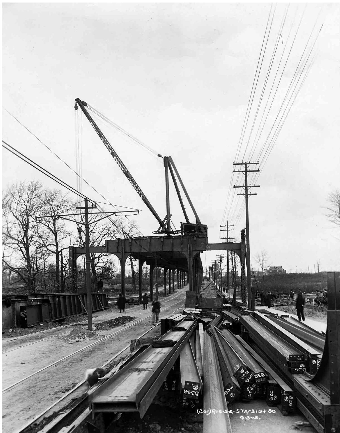
It is now April 3, 1915 and we are looking northeast along Jerome Avenue towards the north end of the under-construction Mosholu Parkway Station. The trolley poles of the Union Railway's Jerome Avenue Line will soon give way to trolley wire ducts attached to the underside of the elevated structure. Granville W. Pullis/PSC photo
