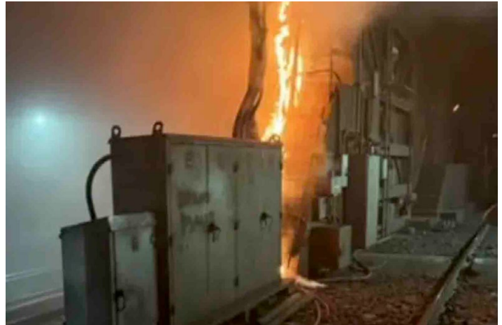
The fire on May 15 in C Interlocking. MTA photo
