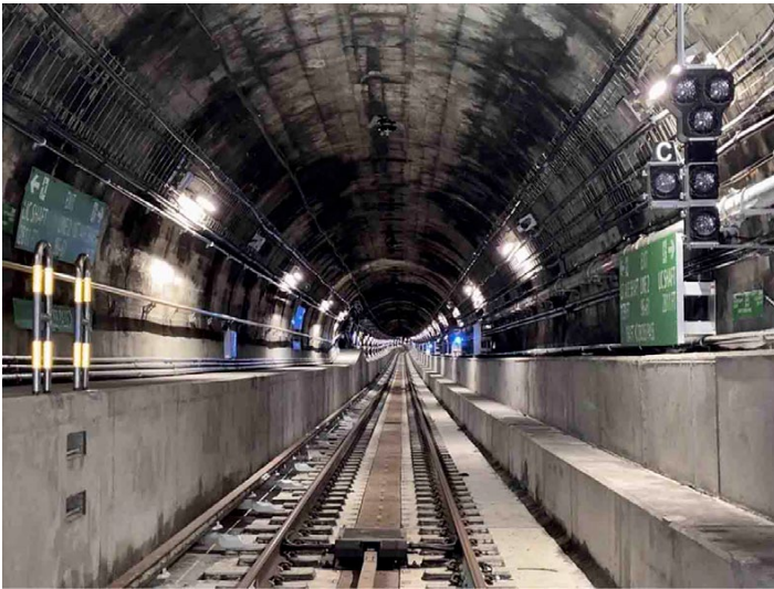
A very recent view looking railroad-west in Line 2 at what we believe to be newly-installed Home Signal No. 582W, which is located at a new control point, CP Low. If this is, in fact, that location it is under the East River and is 1,045 feet east of First Avenue. Amtrak photo
