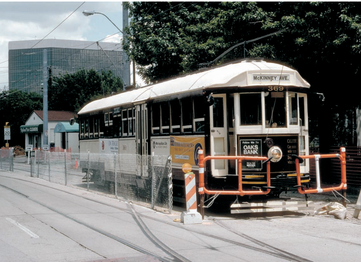
Above, the McKinney Avenue Transit Authority's ex-Melbourne tram negotiates the single track section of line during track reconstruction. Spring-loaded gates are provided to deter motorists from driving onto the tracks where trolleys are operating against the temporary one-way traffic flow.
